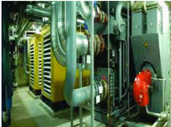
Beijing has its own strategy for supplying clean and efficient energy systems, such as a trigeneration system here at the Beijing Gas Group (Beijing Energy-net De Co Ltd)
